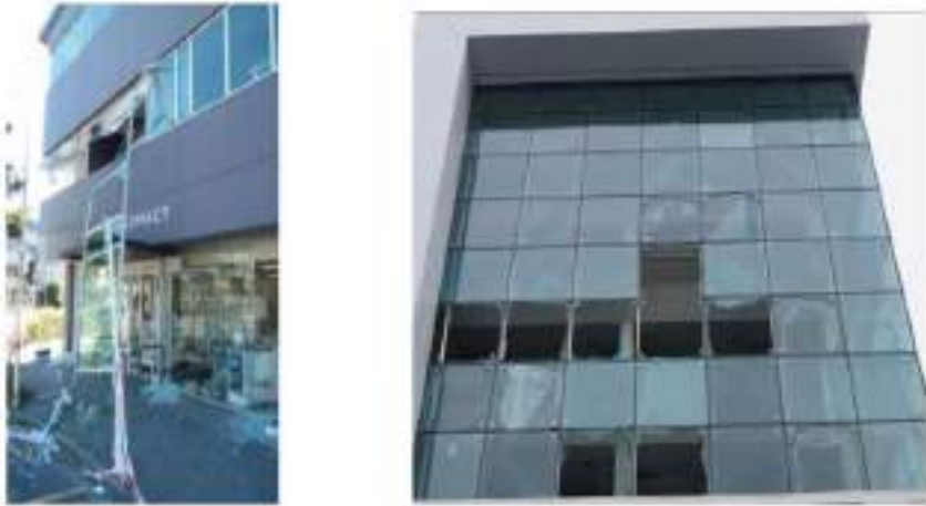
Fig.3 : The falling of aluminum frame because disconnection of cladding (left), The damage of Spider glass after earthquakes in New Zealand buildings (right)
